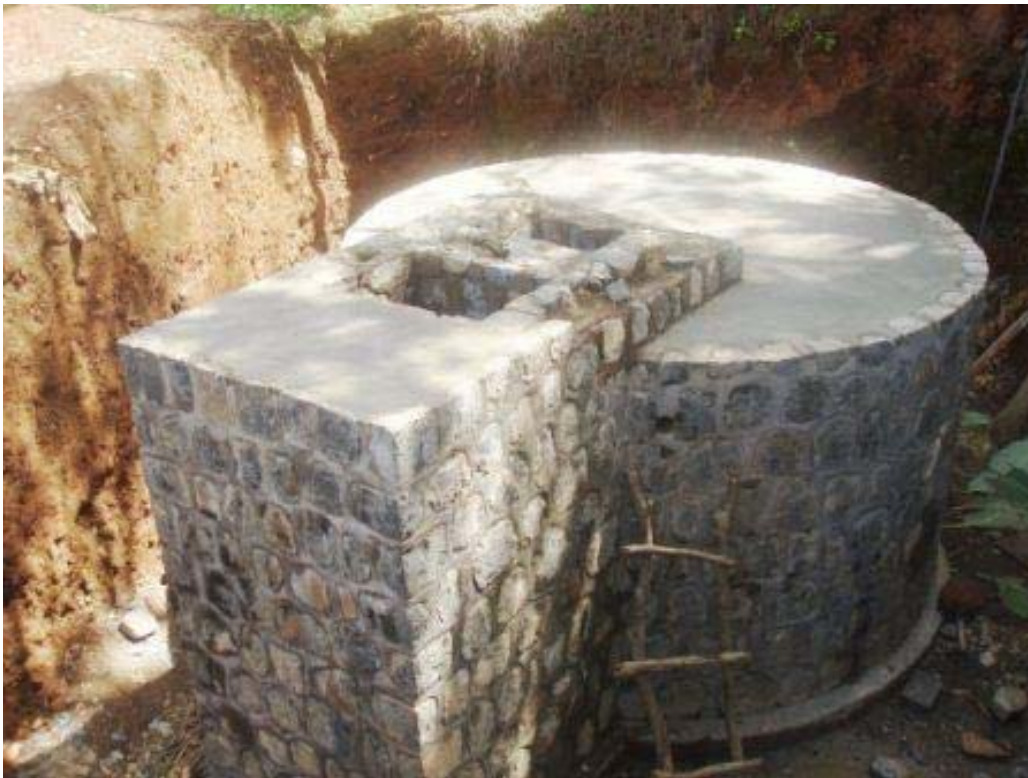
Tank's site view. The ground is dug, the tank built and the surroundings refilled.
