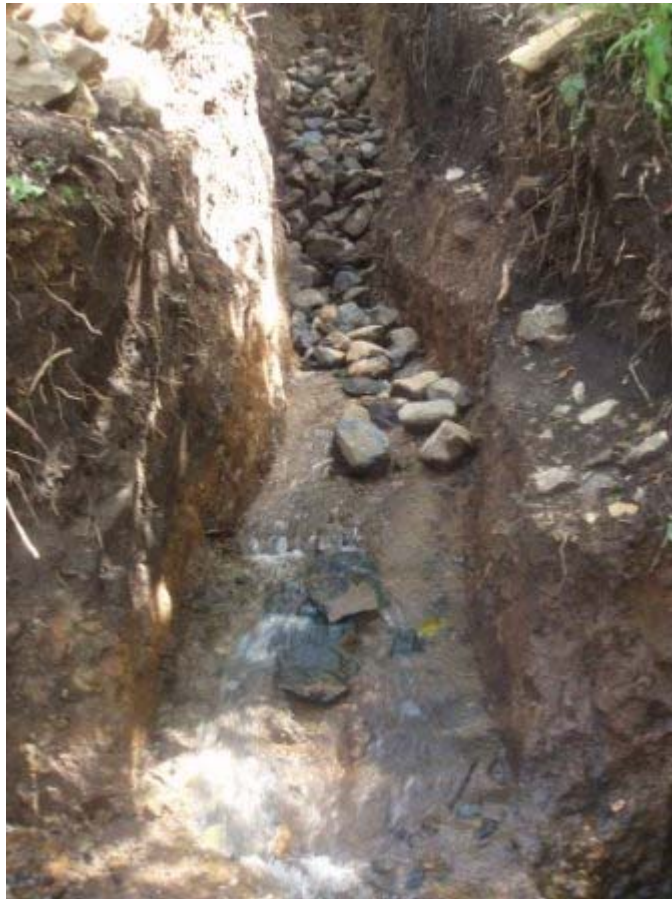
Here, a catchment needs to be built to collect water into the old catchment since more water sources have been identified.
