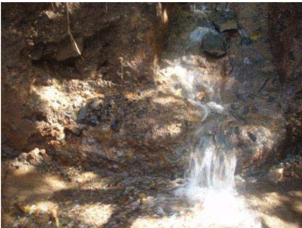
This water sources have been dug and now need construction to channel them into the old catchment
