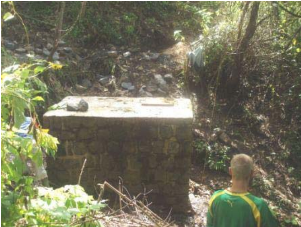
Old spring catchment which needs renovation works
