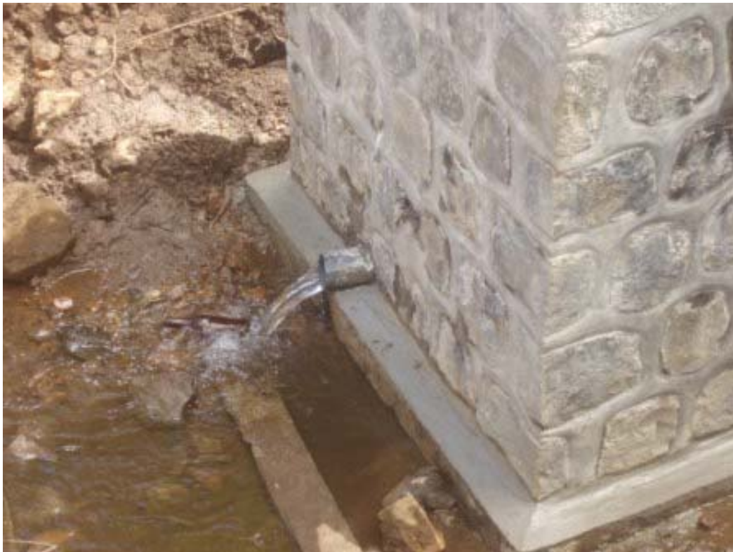
The outlet, which will be channeled into the storage tank from this catchment by pipes
