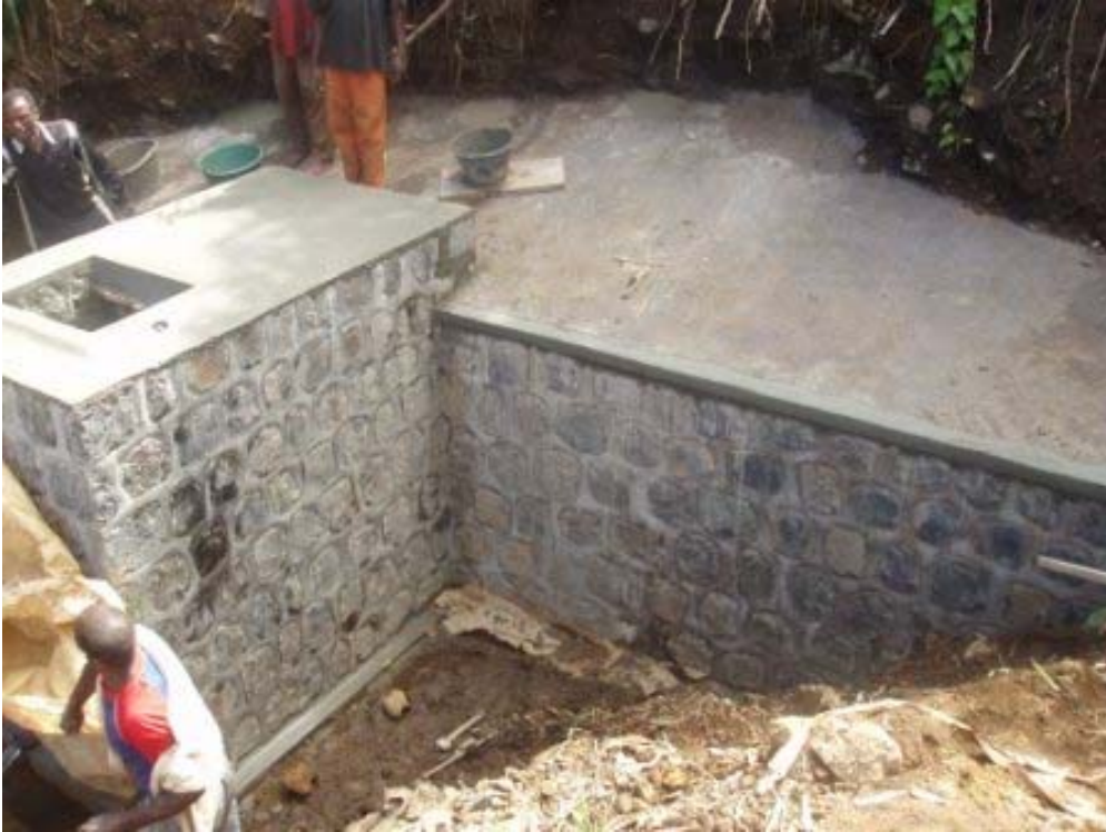
Newly built spring catchment to collect water from the different sources in the ground and channel it into the storage tank for onwards distribution
